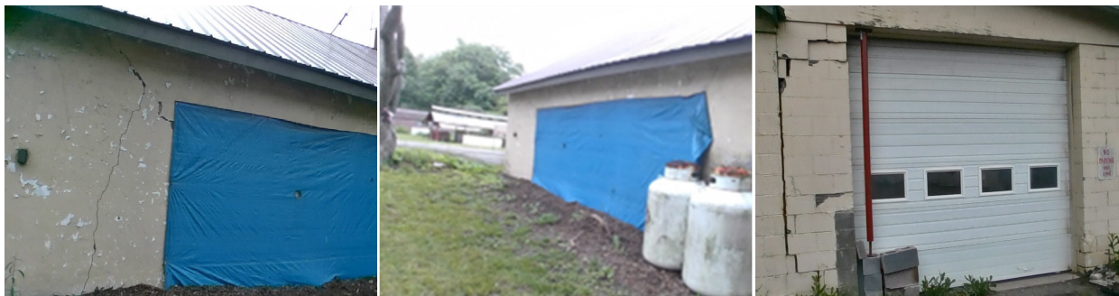
Tarp Covering Damage From 2019 Automobile Collision
