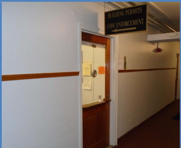
Signs at department offices lacked raised lettering and Braille and were not mounted on the latch side of the door.
