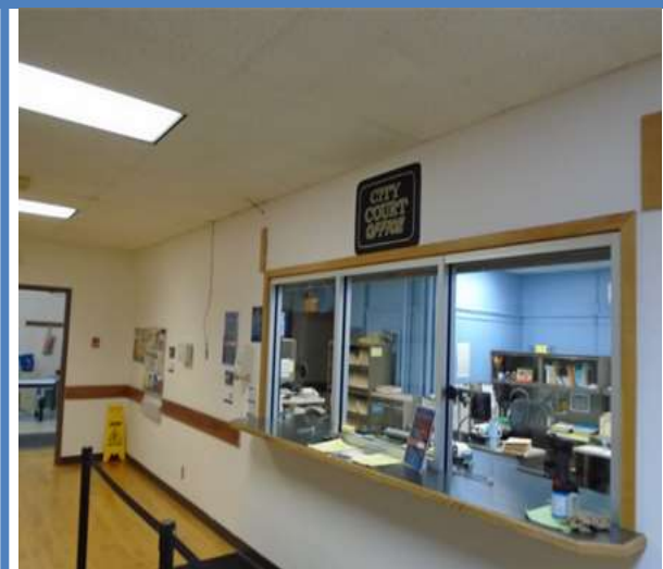
Service counter without an accessible portion no higher than 36 inches at the City Court.
