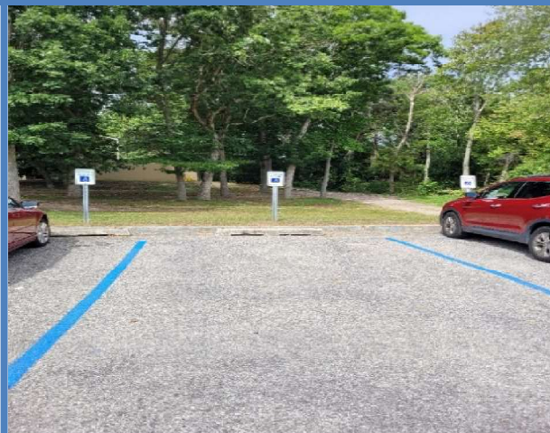
Parking spaces marked accessible but with no access aisles at the Senior Center.
