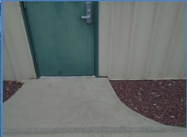
Not enough clearance on the latch side of the door to accommodate a wheelchair at the Recycling Center.
