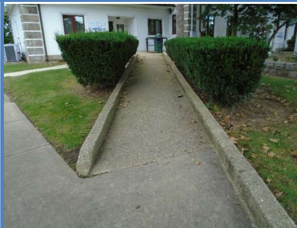
Access ramp with no railings at the approach to the Parks Department.
