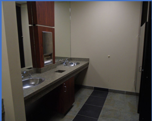
The first-floor restrooms in City Hall do not have at least 60 inches diameter of clear floor space available for a person in a wheelchair to turn around.
