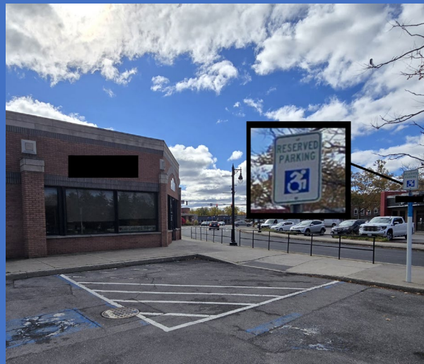
There are no signs identifying van accessible parking spaces at City Hall.
