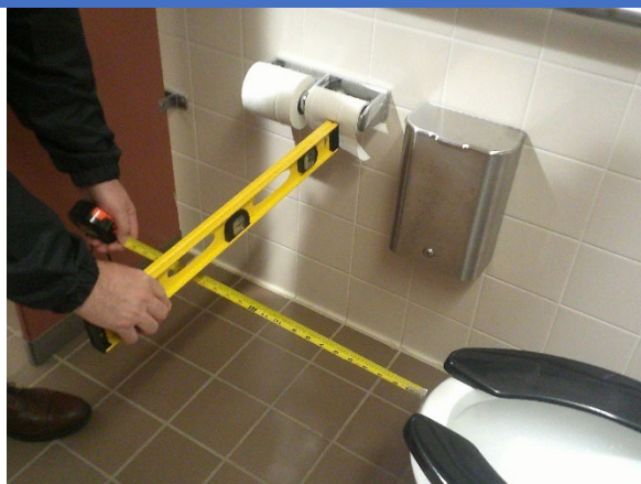
Distance from toilet paper dispenser to front of toilet in Community Center women's restroom is more than ADA guidelines stipulate.
