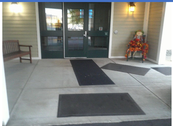
Edges of mats are not secure to the floor at the Town Hall entrance.
