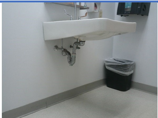
Pipes under the restroom lavatory in Town Hall are not covered or insulated to prevent injury from contact with hot or cold pipes, as well as sharp or abrasive surfaces.
