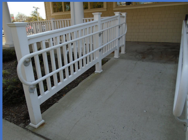
Access ramp at the Senior Center without a curb or barrier to prevent wheelchair castors and/or crutch tips from falling off.
