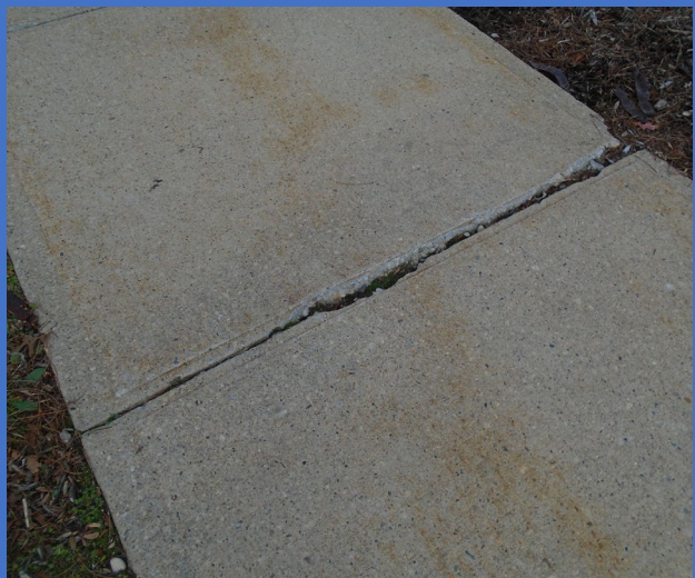
An opening in the pavement along the accessible route to Town Hall is more than one half inch.
