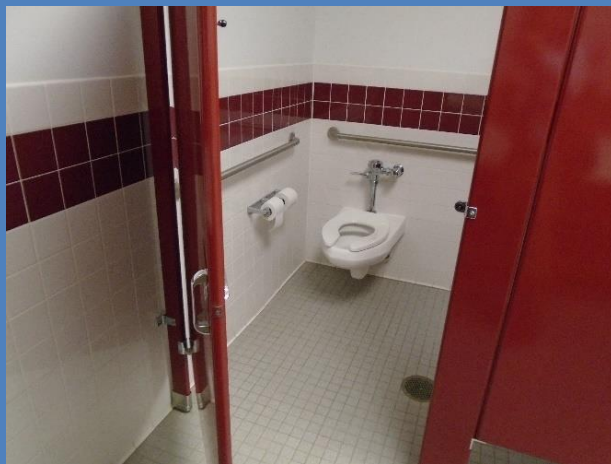
Doors to accessible stalls in restrooms at the Town Hall did not have automatic door closers.
