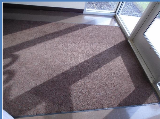
Mat at the DPW building entrance was not securely attached.
