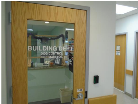
Sign for the Building Department at the Town Hall was not mounted on the latch side of the door with raised letters or Braille.
