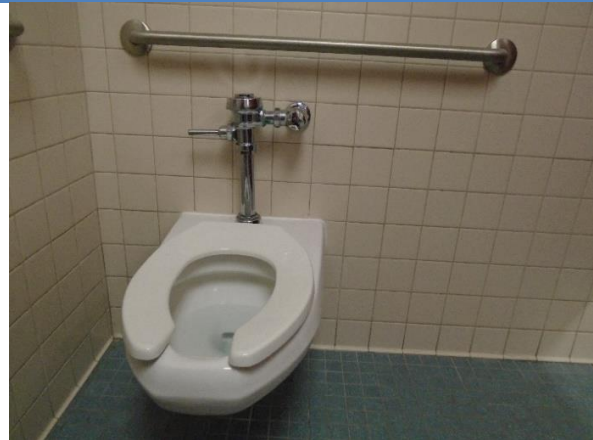
The flush control in the men's restroom at the Town Court was not located on the open side of the water closet.
