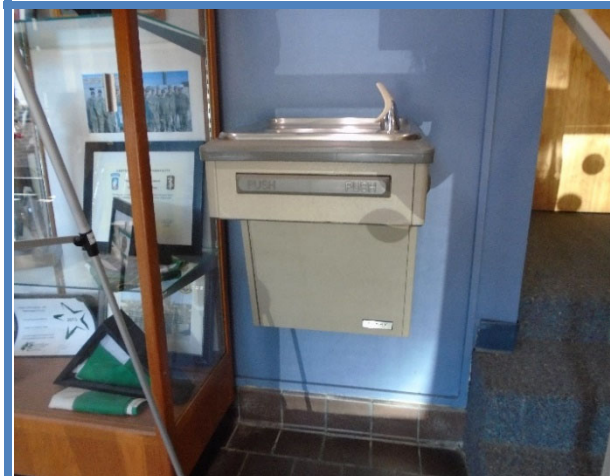
Water fountain mounted too high at the Town Hall.
