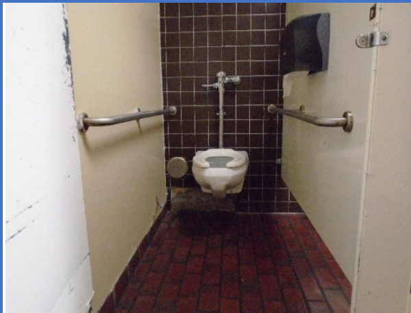
Stall door/stall not wide enough and no rear grab bar in the City Library men's restroom.
