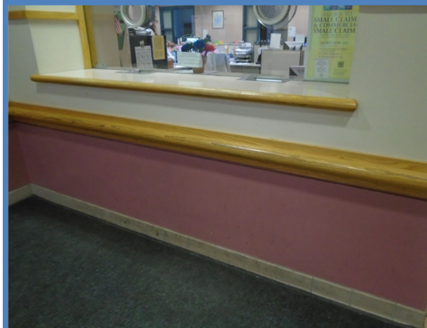
Service counters at the Public Safety Center without an accessible portion no higher than 36 inches.
