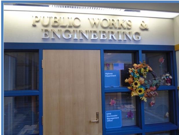
Signs in the Public Operations Center were mounted too high and without raised lettering and Braille.
