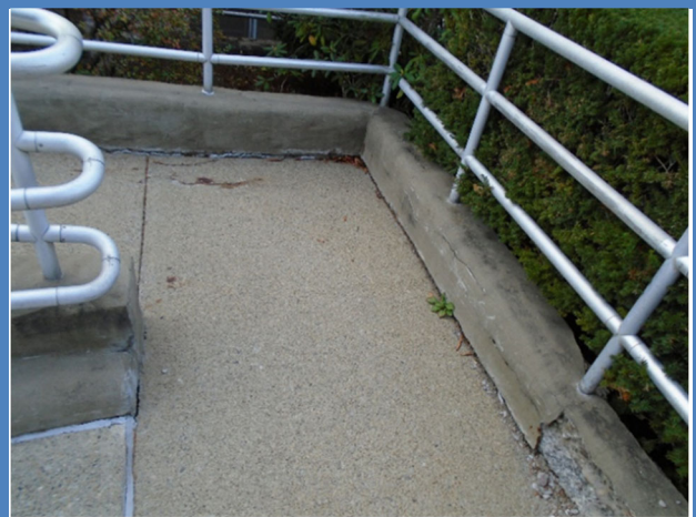
Ramp at the Town Hall main entrance did not have a level landing of at least 60 inches by 60 inches where the ramp changes direction.
