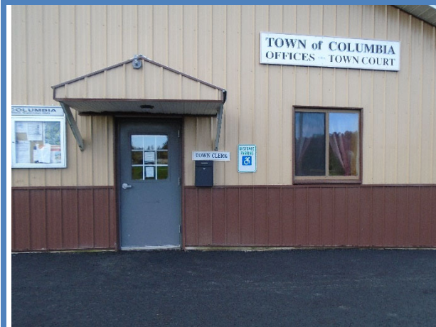
Accessible parking did not have painted lines showing the reserved spots or access aisles.
