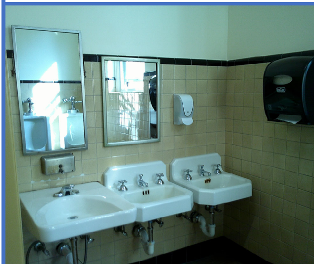
Mirrors, soap dispenser and towel dispenser mounted too high, and pipes under lavatories not insulated to protect against potential injuries from contact with hot or cold pipes, as well as sharp or abrasive surfaces.
