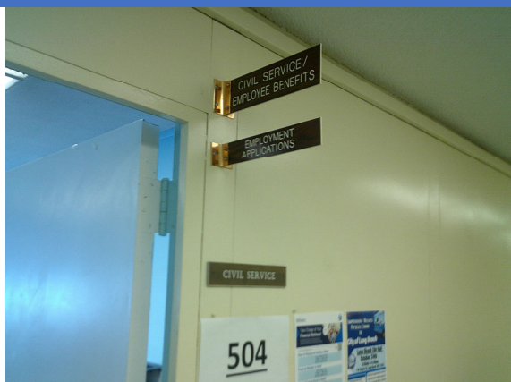
Signs in the City Hall without raised lettering or Braille and not mounted on the latch side of the door.
