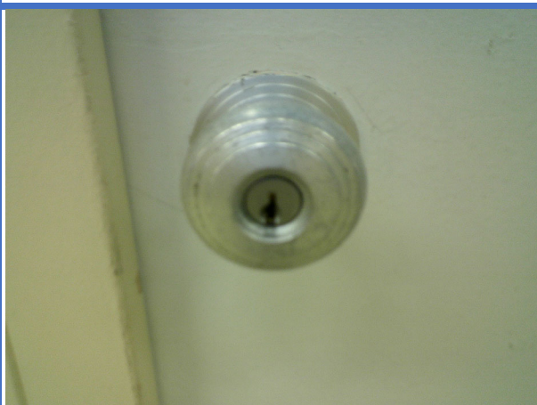
Office doors at City Hall have doorknobs instead of accessible handles such as latches or levers.
