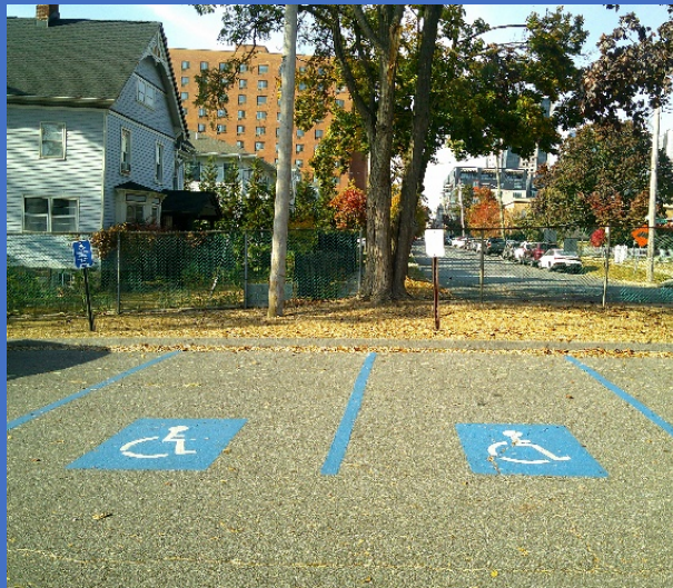
Accessible parking spaces with no signs or access aisles at the Senior Center.
