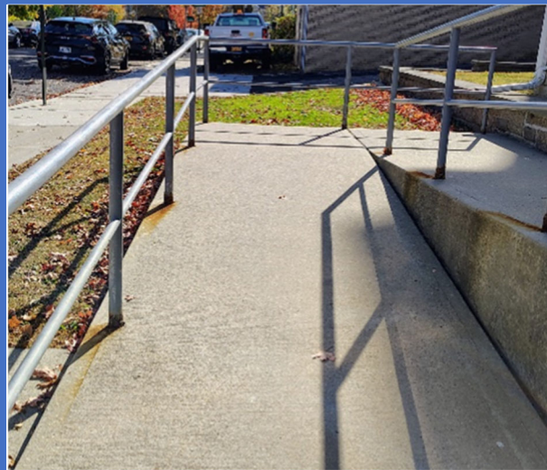
Access ramp to the Fire Department Headquarters does not have handrails on both sides or a curb or other barrier.
