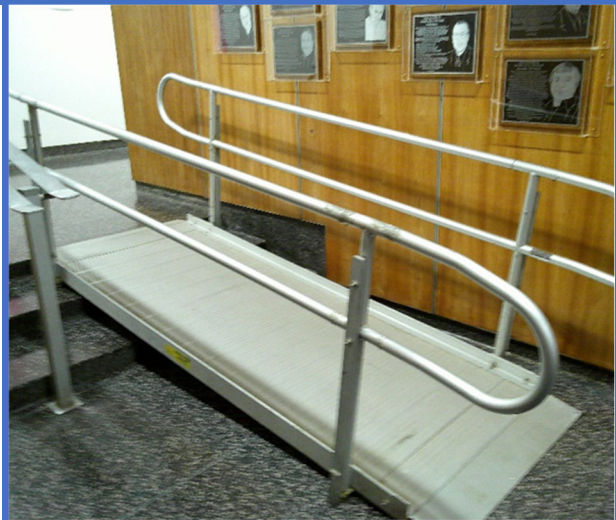
Interior access ramp in City Hall is not properly sloped.
