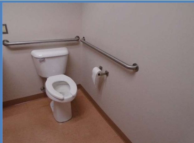
Handrails at the City Court's accessible restroom did not extend far enough and were mounted too high.
