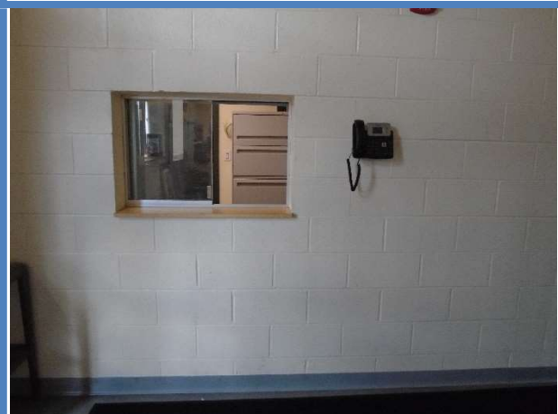
Service counter and call buttons at the Code Enforcement office (Fire Station) are too high.
