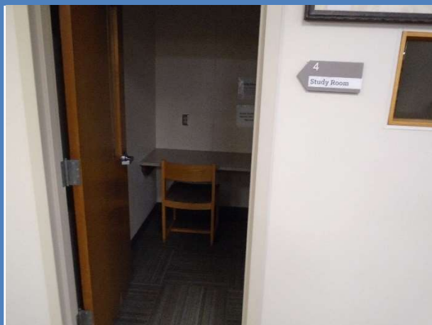
Interior doors to the study rooms at the Public Library with an opening width of less than 32 inches.
