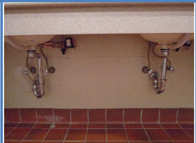
Pipes under lavatories in the Town Court restrooms were not insulated to prevent potential injury from contact with hot or cold pipes, as well as sharp or abrasive surfaces.
