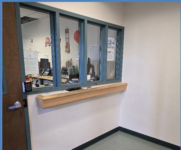
Service counter at the Court Clerk's office without an accessible portion no higher than 36 inches.
