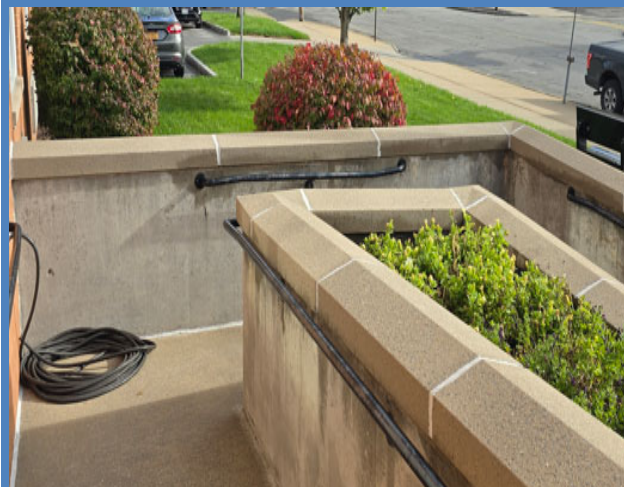
Police Department entrance ramp did not have a level landing where it changes direction that is at least 60 inches by 60 inches and there was a temporary obstruction.
