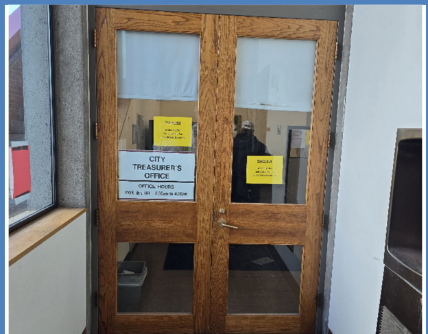
Signs at the entrance to the Treasurer's Office in City Hall without raised lettering and Braille.
