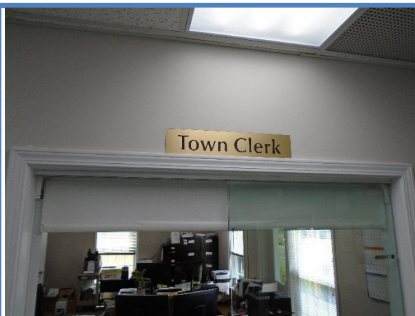
Sign without raised lettering and Braille and not mounted on the latch side of the door at the Town Clerk's office.
