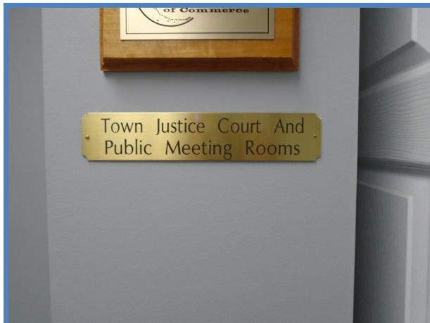
Sign without raised lettering and Braille and not mounted on the latch side of the door at the Town Court and public meeting rooms.
