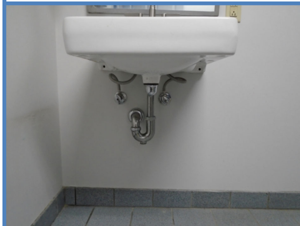
Pipes under restroom lavatories in the men's restroom were not insulated to protect against potential injuries from contact with hot or cold pipes, as well as sharp or abrasive surfaces.
