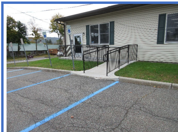
Parking spaces without marked access aisles, and blocking accessible entrance at the Senior Center/Library.
