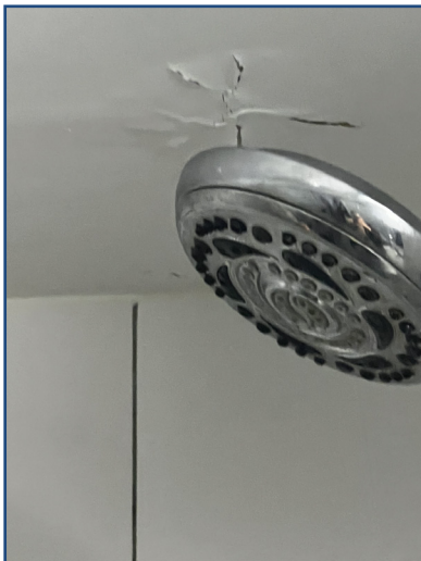
Hour Children - Eclipse – bathroom shower ceiling water leak
