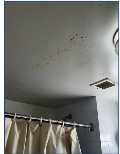
CAMBA – bathroom ceiling water leak
