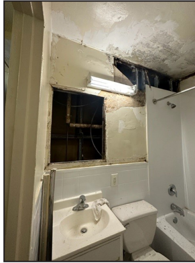
Figure 5 - Holes in a bathroom wall in a North Shore townhouse.
