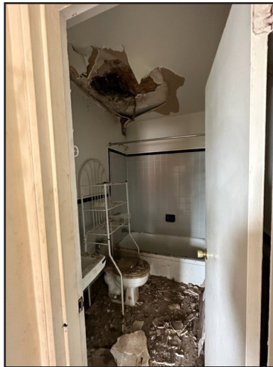
Figure 2 - Collapsed ceiling in a bathroom of an Arverne unit.
