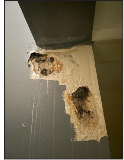
Figure 6 - Mold on the wall in a North Shore townhouse.
