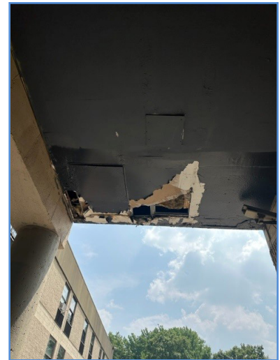
Figure 9 – Deteriorating ceiling in Building 55.
