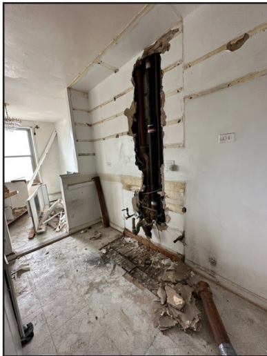
Figure 1 - Collapsed wall in kitchen of an Arverne unit.
