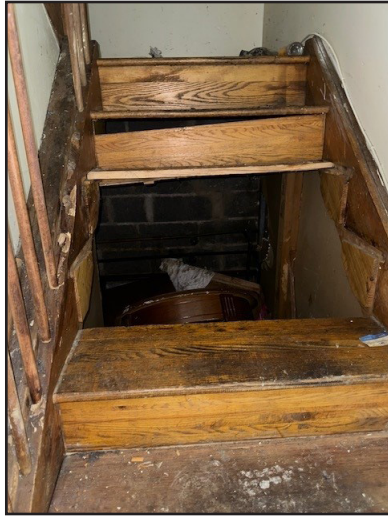
Figure 4 - Missing steps in a North Shore townhouse.
